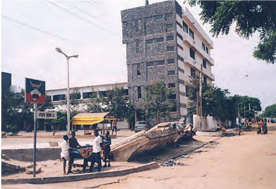
Photo 9: Picture showing the 1998 broken walls of LCI headquarters in Korle-Gonno (Credit: Marleen de Witte, 1998).
